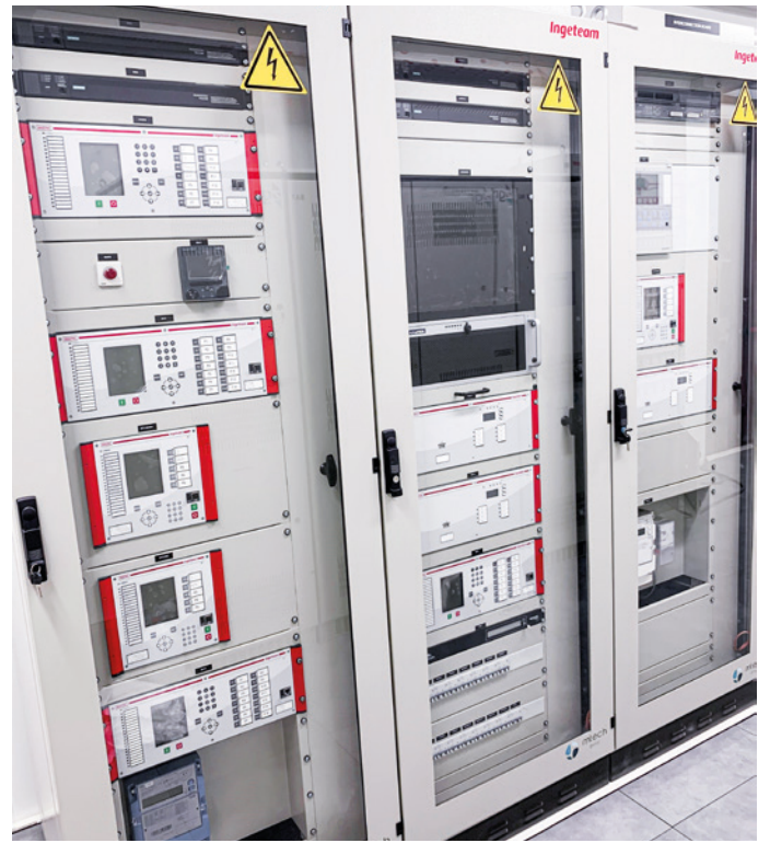
Protection and control system cabinets
