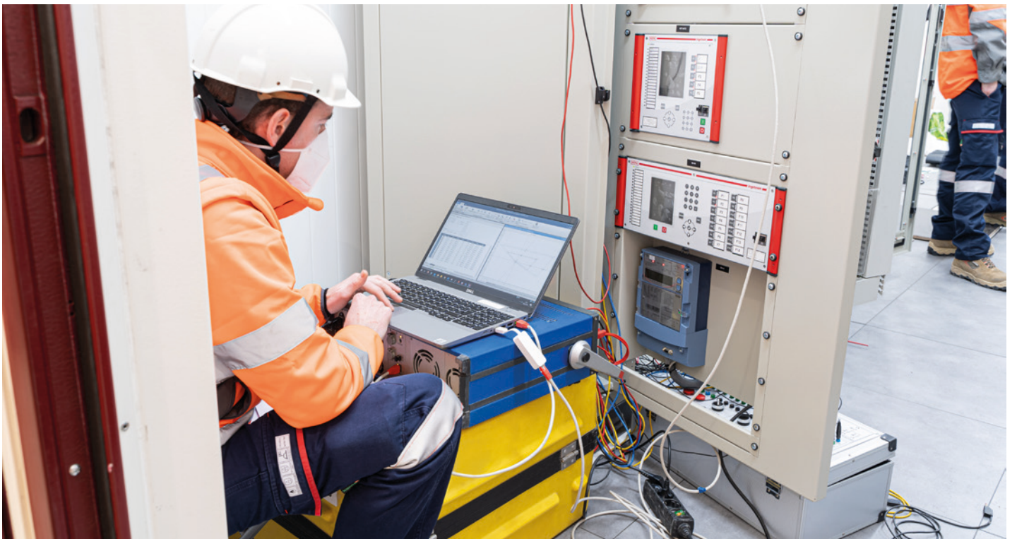
Protection devices test
