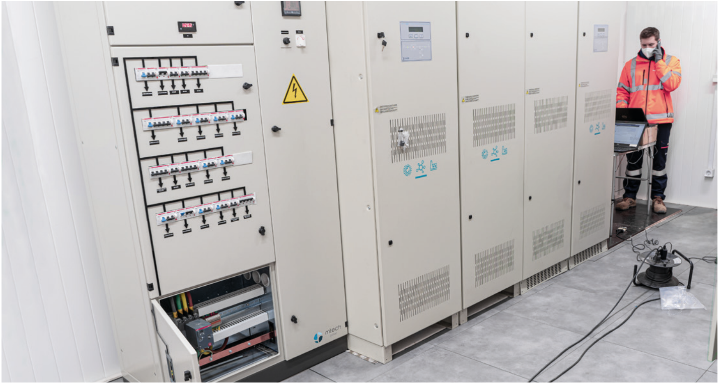
Remote control test
