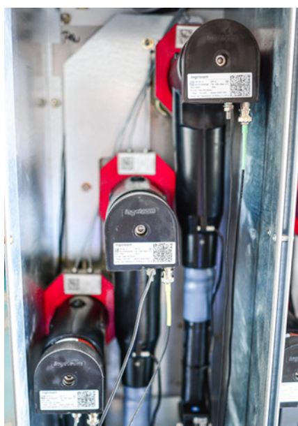
INGEPAC™ SR GR in cabinet
