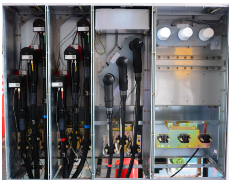
INGEPAC™ SR GR installed in cells
